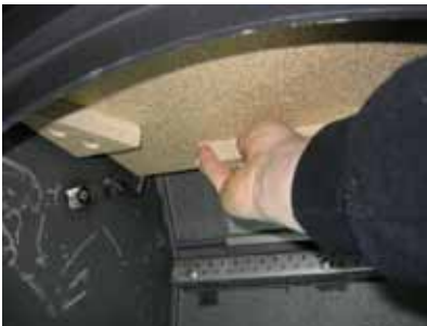
e. The upper baffleplate is removed from the brackets and lifted out of the fire-chamber
