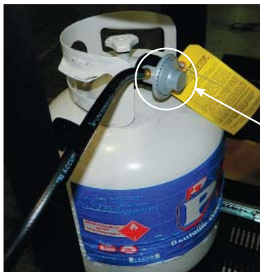
Gas connection @ tank
