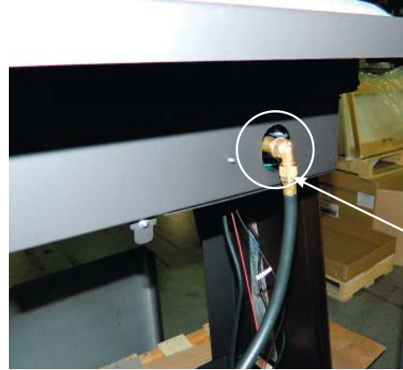
Gas connection @ unit
