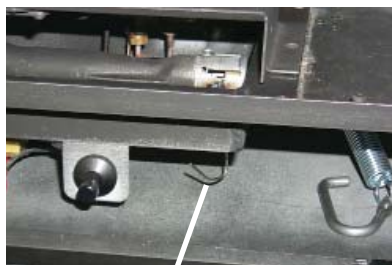
Aeration Adjustment Wire
